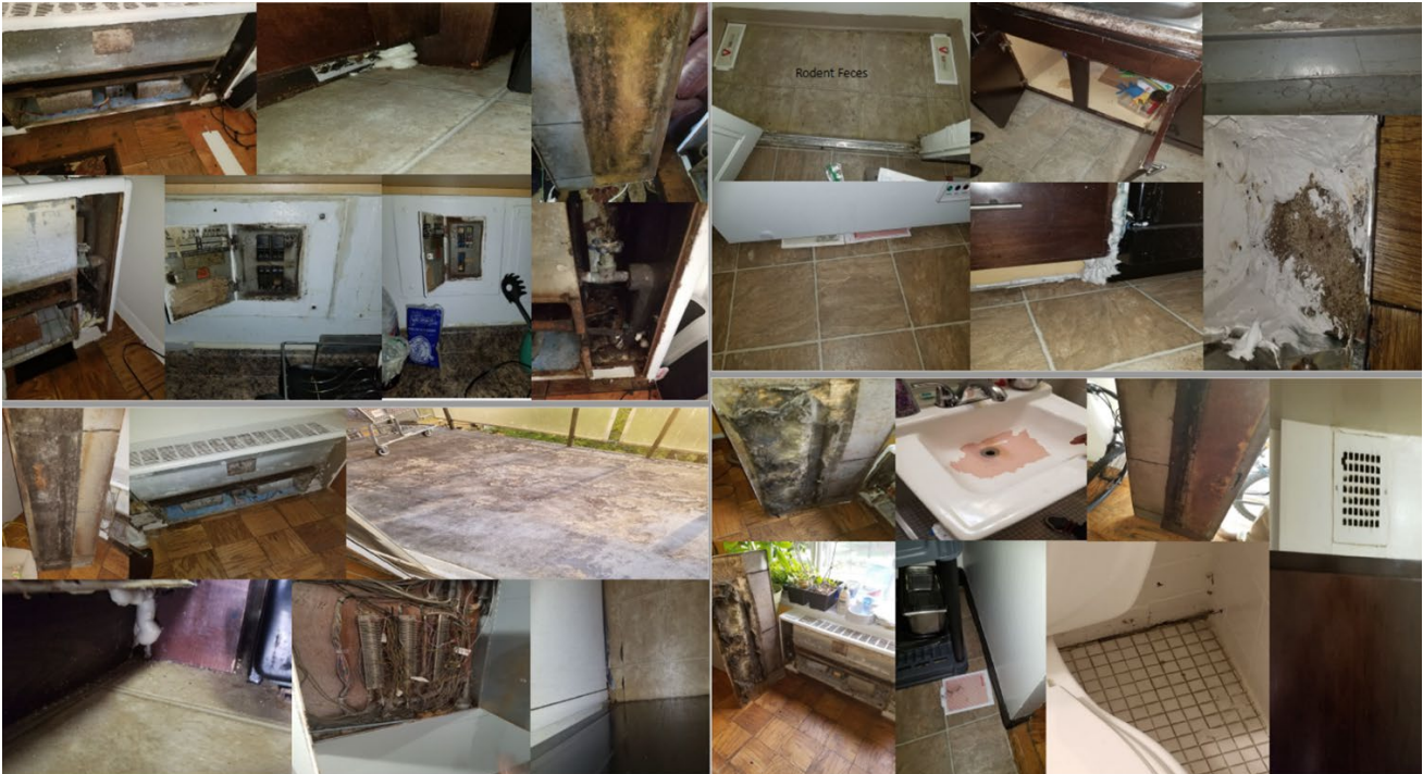
Figure 1 – Pictures of conditions in multiple units at Serrano Apartments from NAACP Letter to Arlington County dated April 30, 2021
