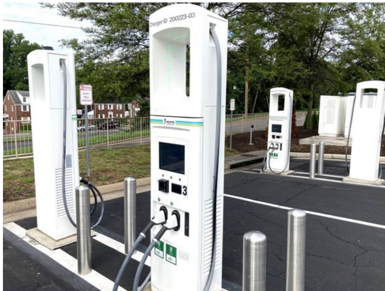
An electric vehicle charging station
