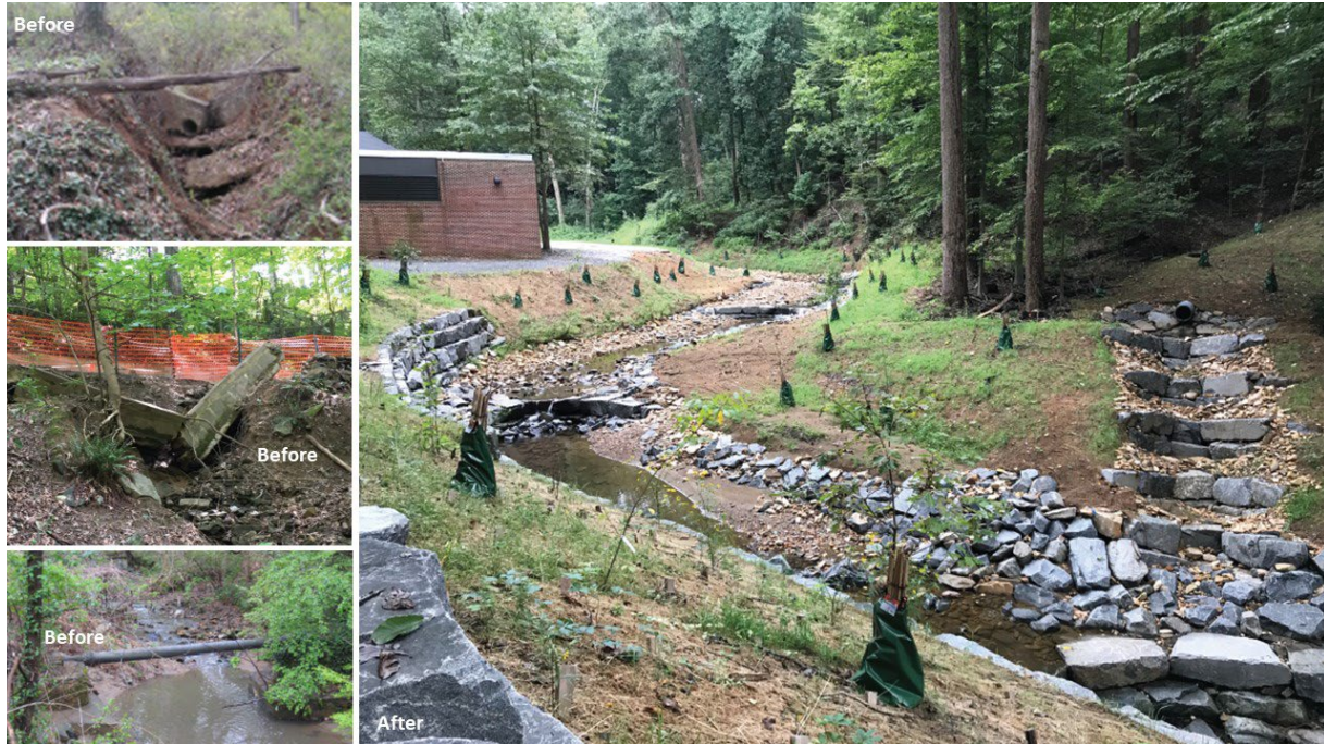
Windy Run before and after the 2018 stream resiliency project. Before: Broken stormwater infrastructure, erosion undermining the trail, vulnerable sanitary sewer pipe. After: Stable, wide channel and gently sloping banks. Stone structures protect infrastructure and prevent future erosion.
