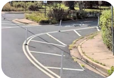
Tactical projects - quick interventions. (Pictured: curb extension via paint and bollards at Yorktown Blvd. & N. George Mason Dr.)
