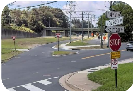
Construction projects. (Pictured: intersection of Fairfax Dr., 14th St. and Queen St., where the County installed sidewalks and improved ramps)
