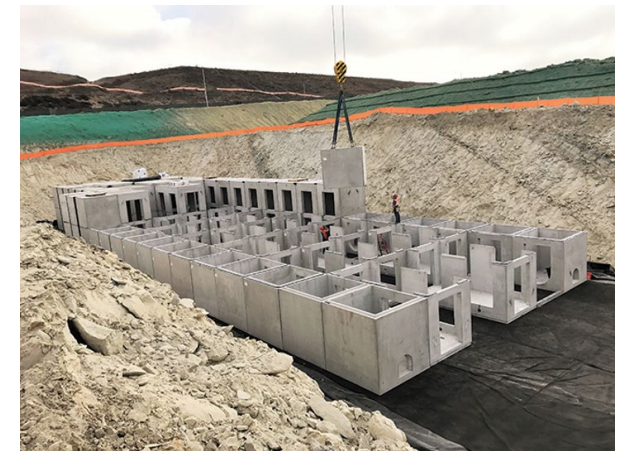
Example of stormwater detention vault, credit: Oldcastle infrastructure
