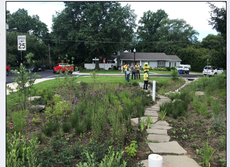
Walter Reed Dr / 5 th Street S ($1.1m) Intersection and bioretention completed fall 2021
