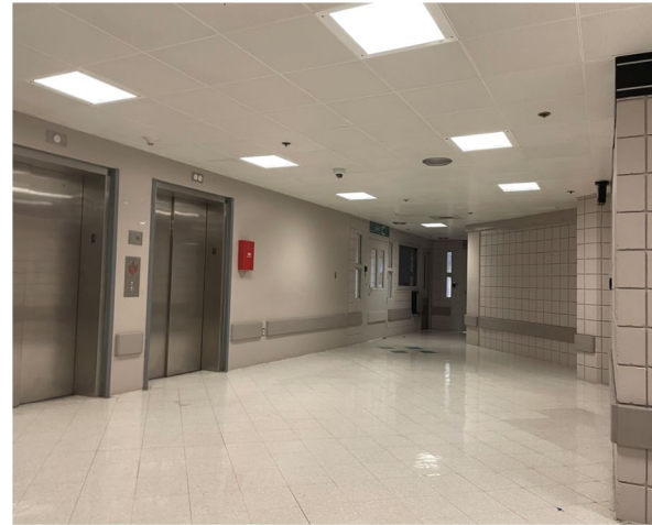
Existing T8 Fluorescent Lighting for Retrofit at the Courts/Police and Detention Center
