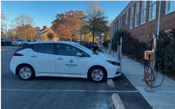
Public and County Fleet EVSE
