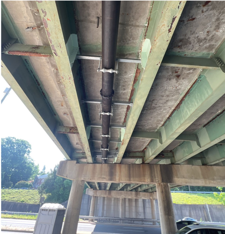
12" water main under N. Rhodes/ Queen St Bridge over Route 50 in Fort Myer Heights
