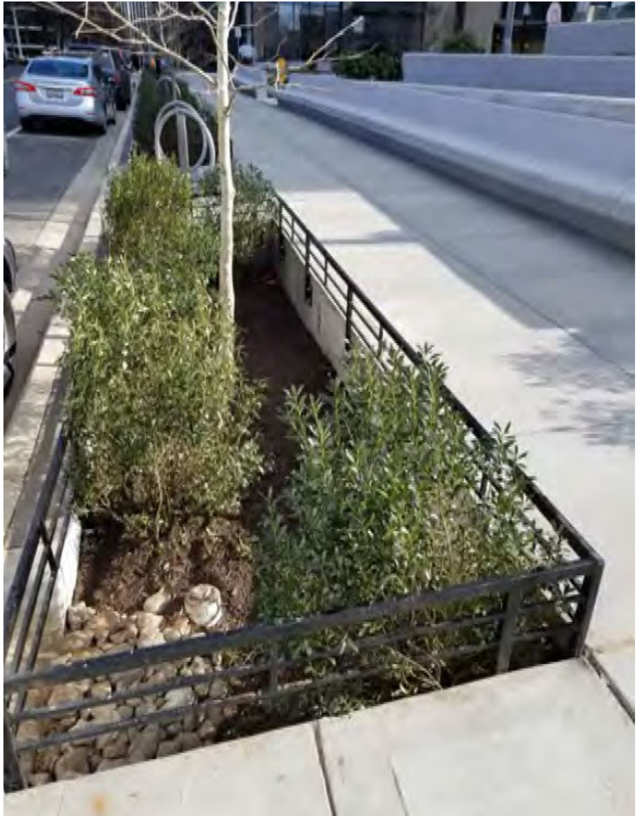
Tree Filter #1: Overall completed tree filter facility with plants, mulch, and splash rocks installed.
