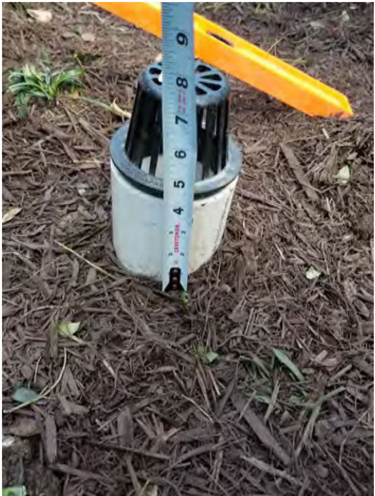
Tree Filter #3: Top of mulch to crest of overflow pipe, Ponding Depth = 5"
