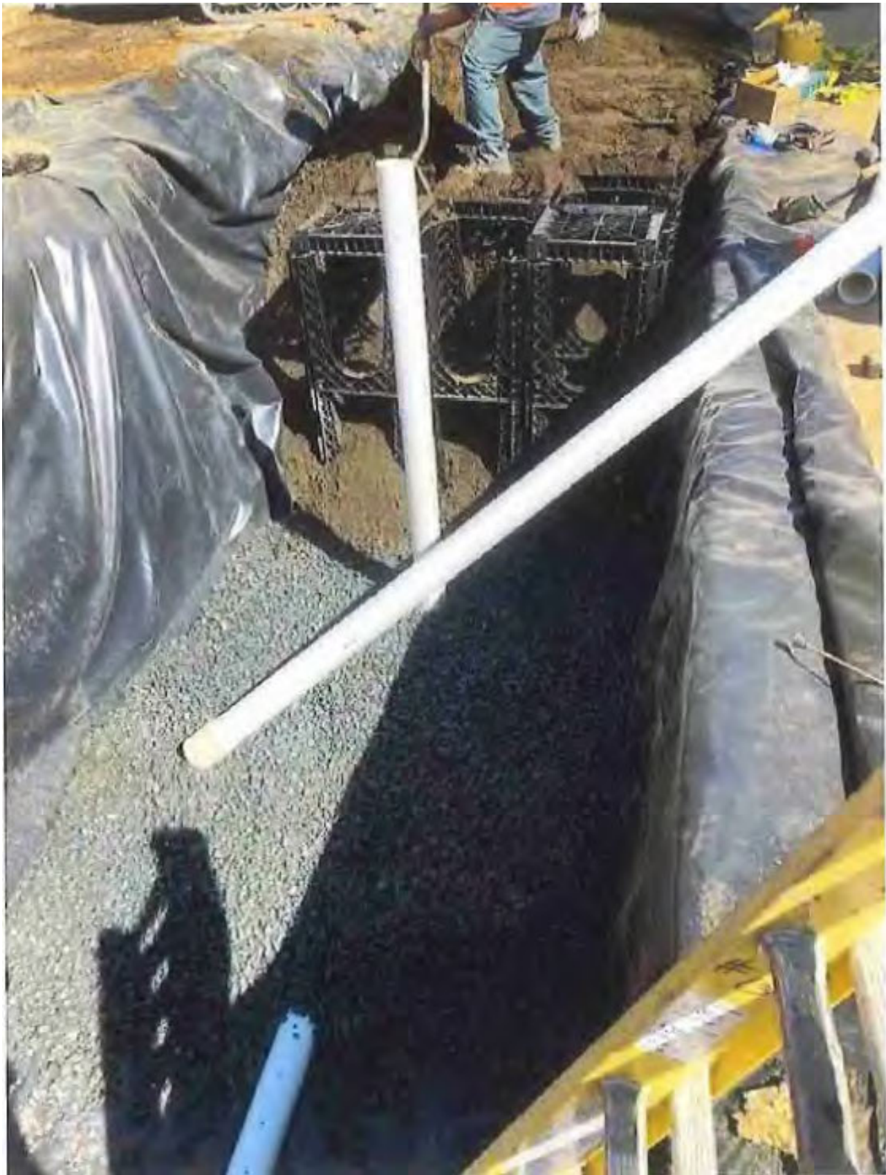
Tree Filter #2: Installation impermeable liner, perforated underdrain pipe, and solid vertical overflow pipe
