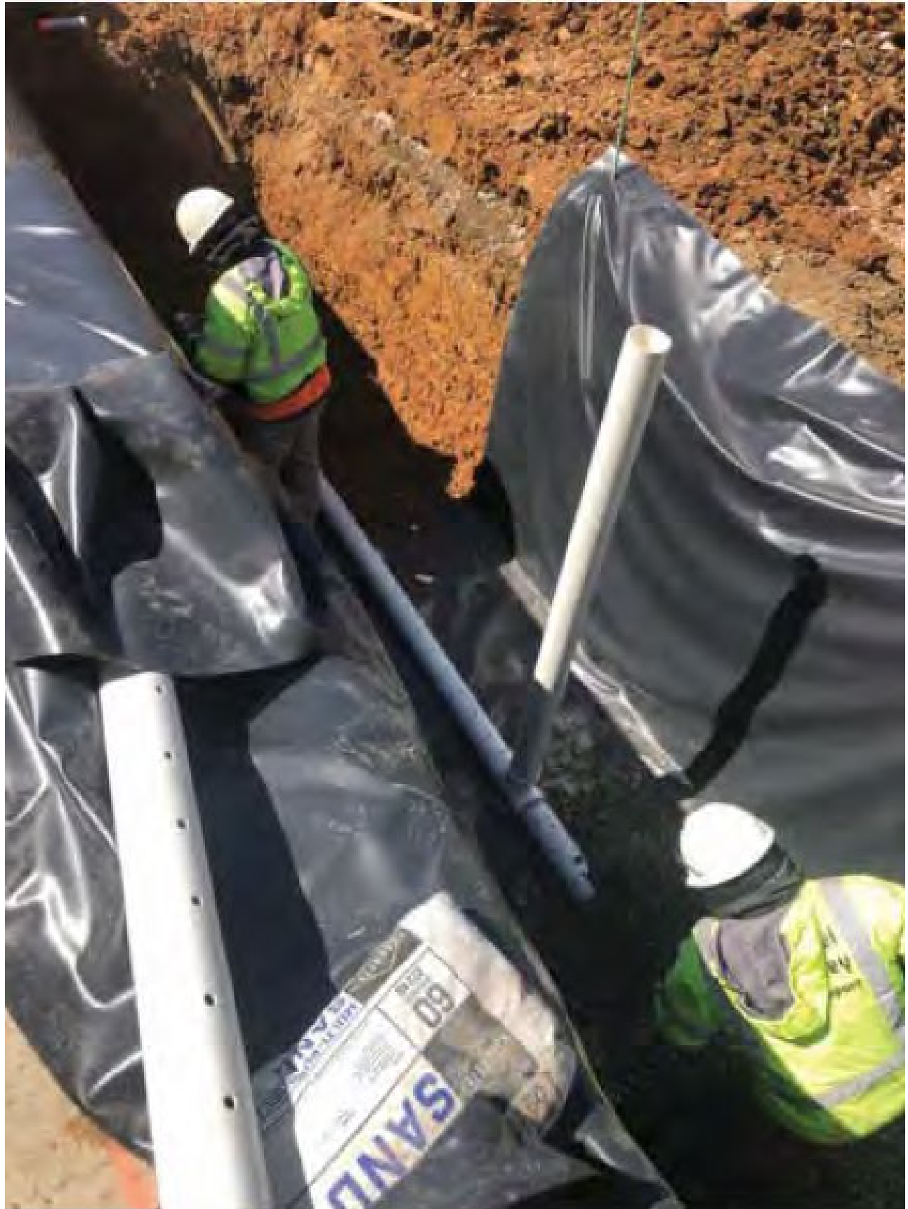
Tree Filter #1: Installation of perforated underdrain pipe and solid vertical overflow pipe
