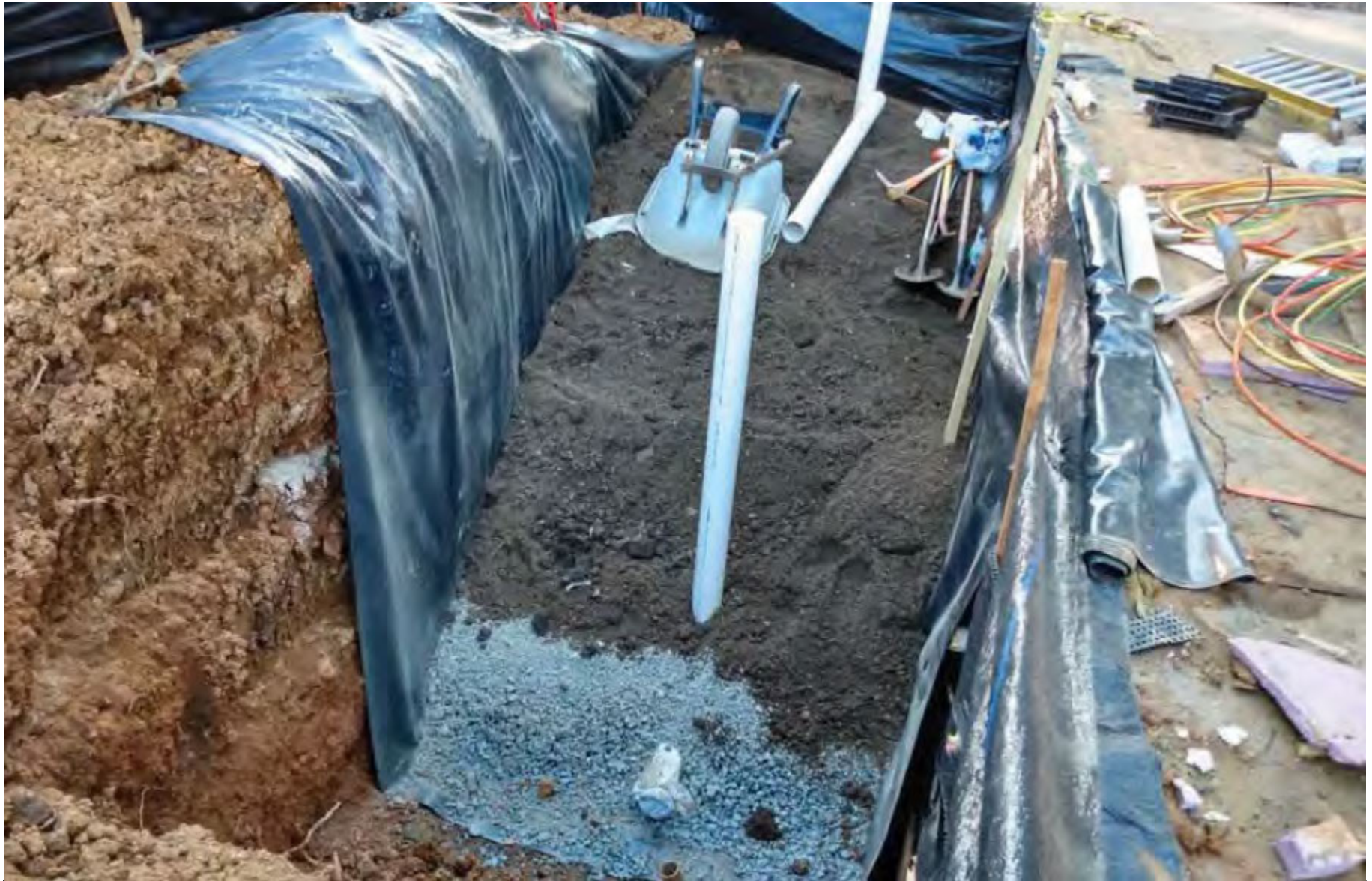
Tree Filter #3: Installation impermeable liner, perforated underdrain pipe, and solid vertical overflow pipe
