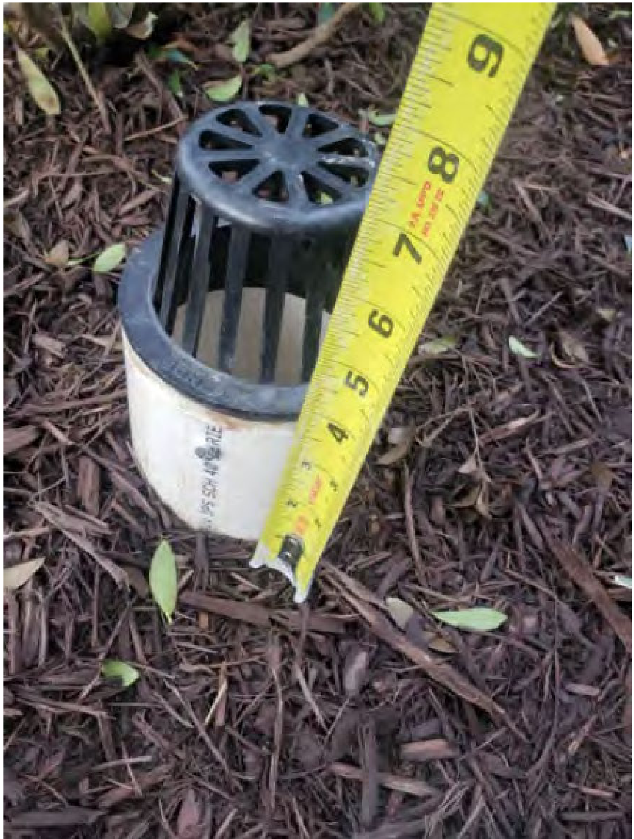
Tree Filter #1: Top of mulch to crest of overflow pipe, Ponding Depth = 4"
