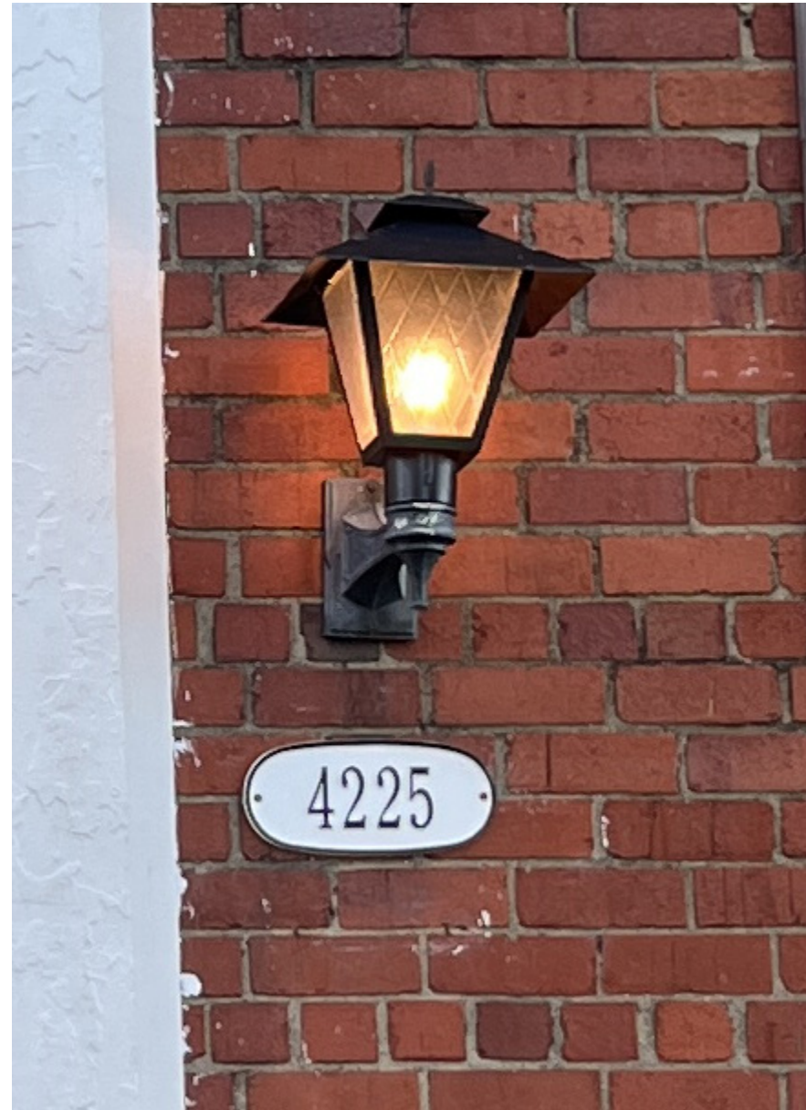
/ EXISTING LIGHT FIXTURE
