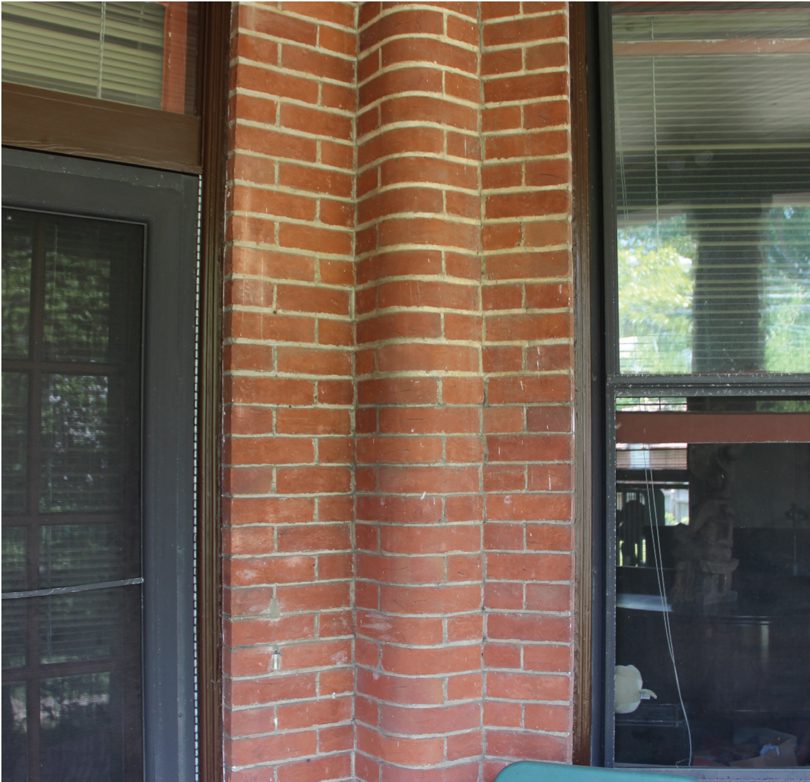
Figure 13: Detail of bullnose radial brick at 3500 14th St. N. looking south. Source: Arlington County Historic Preservation Program, 2016.
