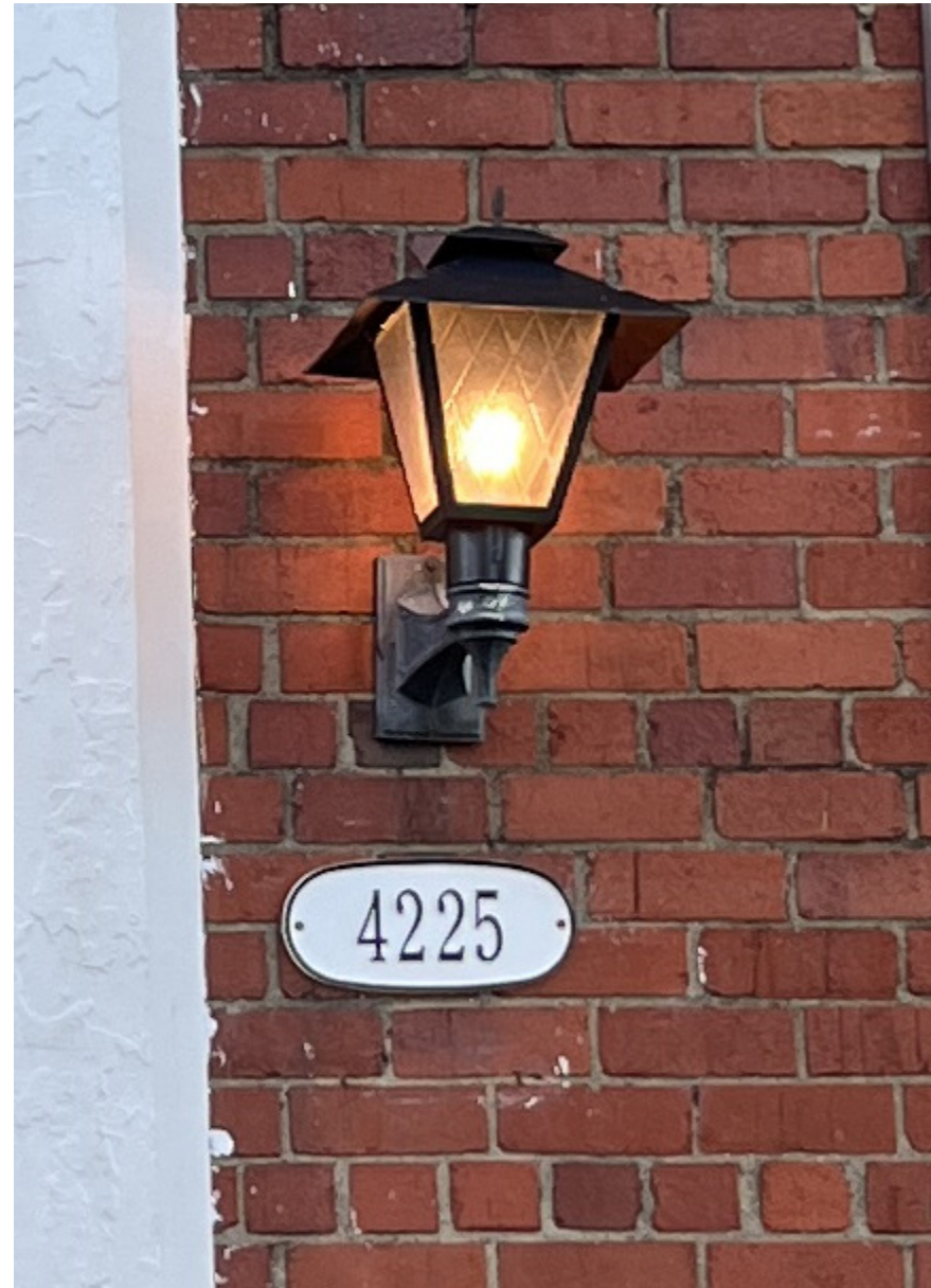
/ EXISTING LIGHT FIXTURE
