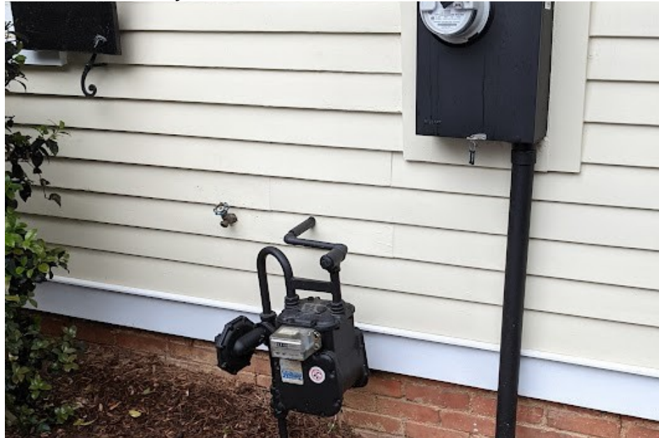
Faucet 1: driveway side
