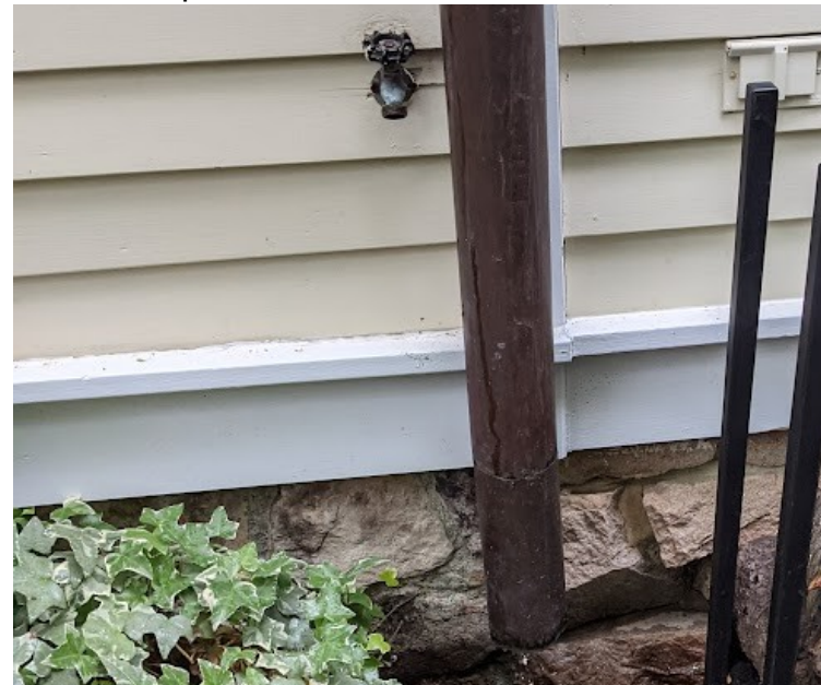
Faucet 2: patio side
