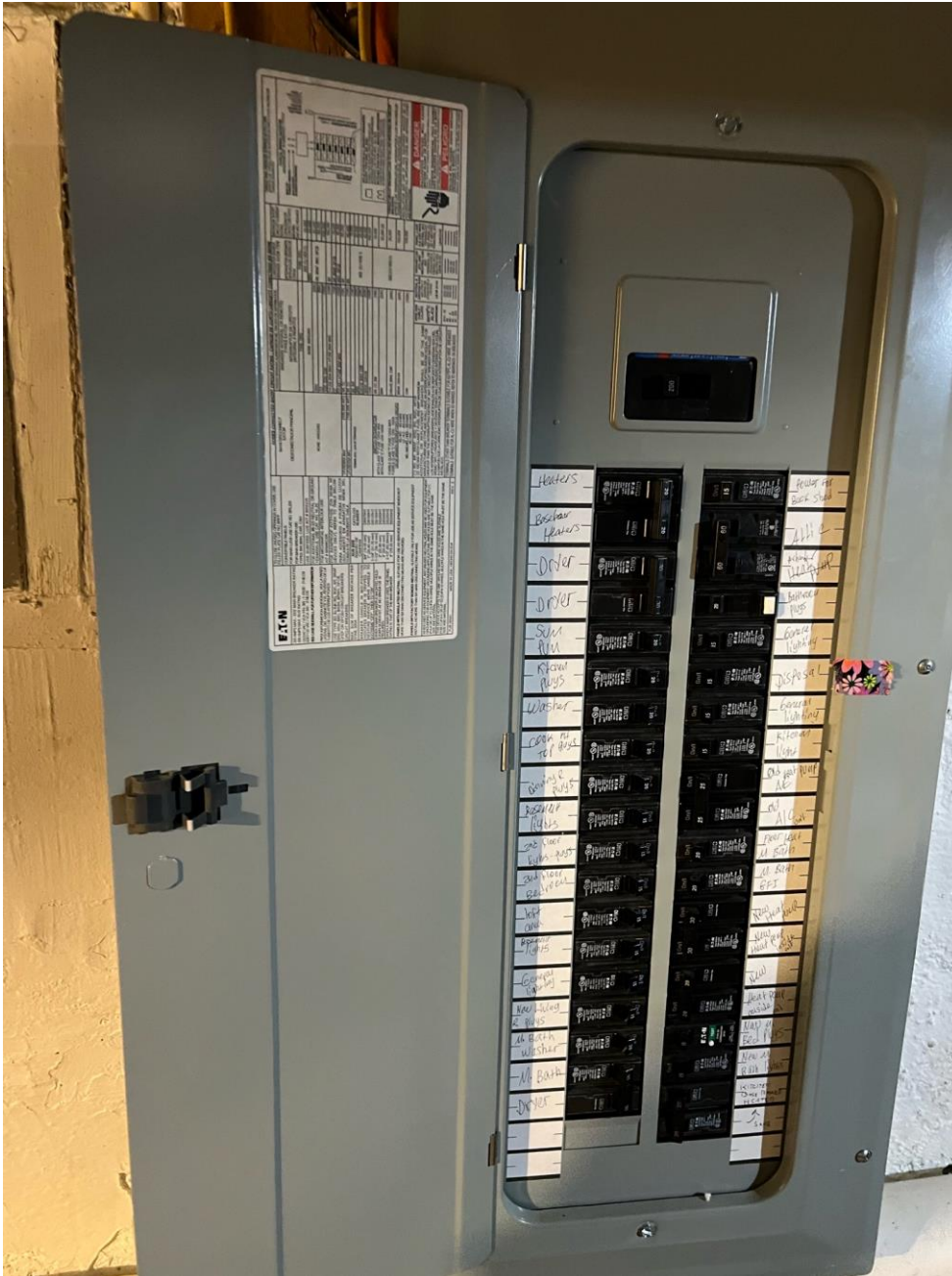
Figure 7: This is a Main Service Panel (MSP). MSP is mounted inside the house.
