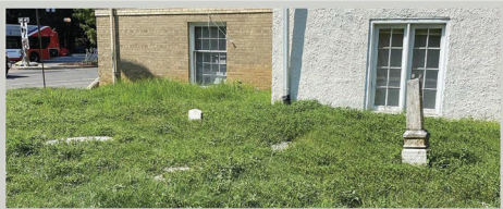
Burial Ground conditions in 2021 prior to the demolition of the 1923 church building. (Courtesy of KCM Group)
