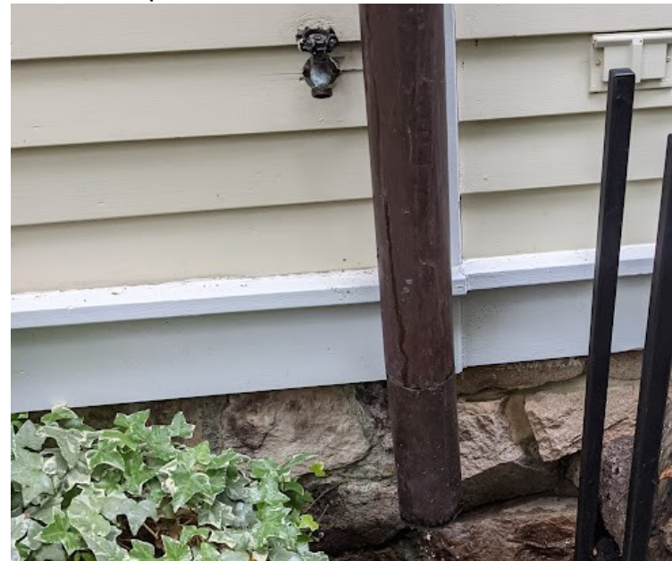
Faucet 2: patio side
