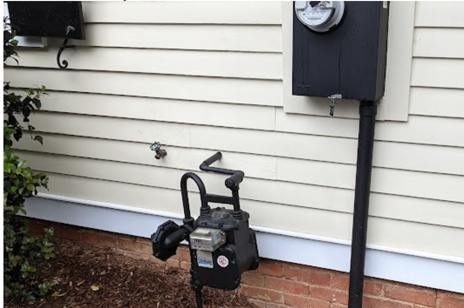
Faucet 1: driveway side
