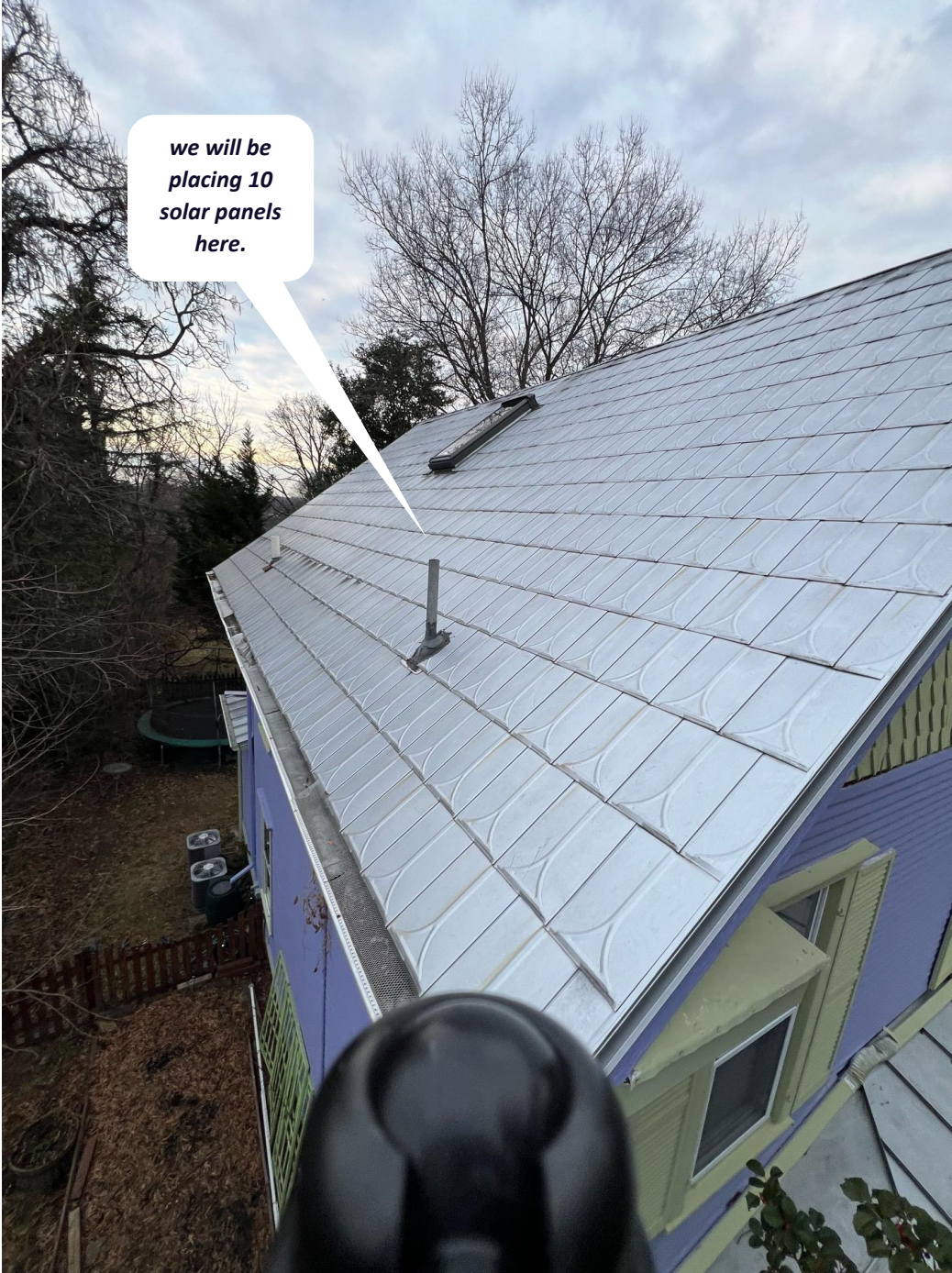
Figure 1: We will be placing total 22 solar panels on the roof. This is the left side of house.
