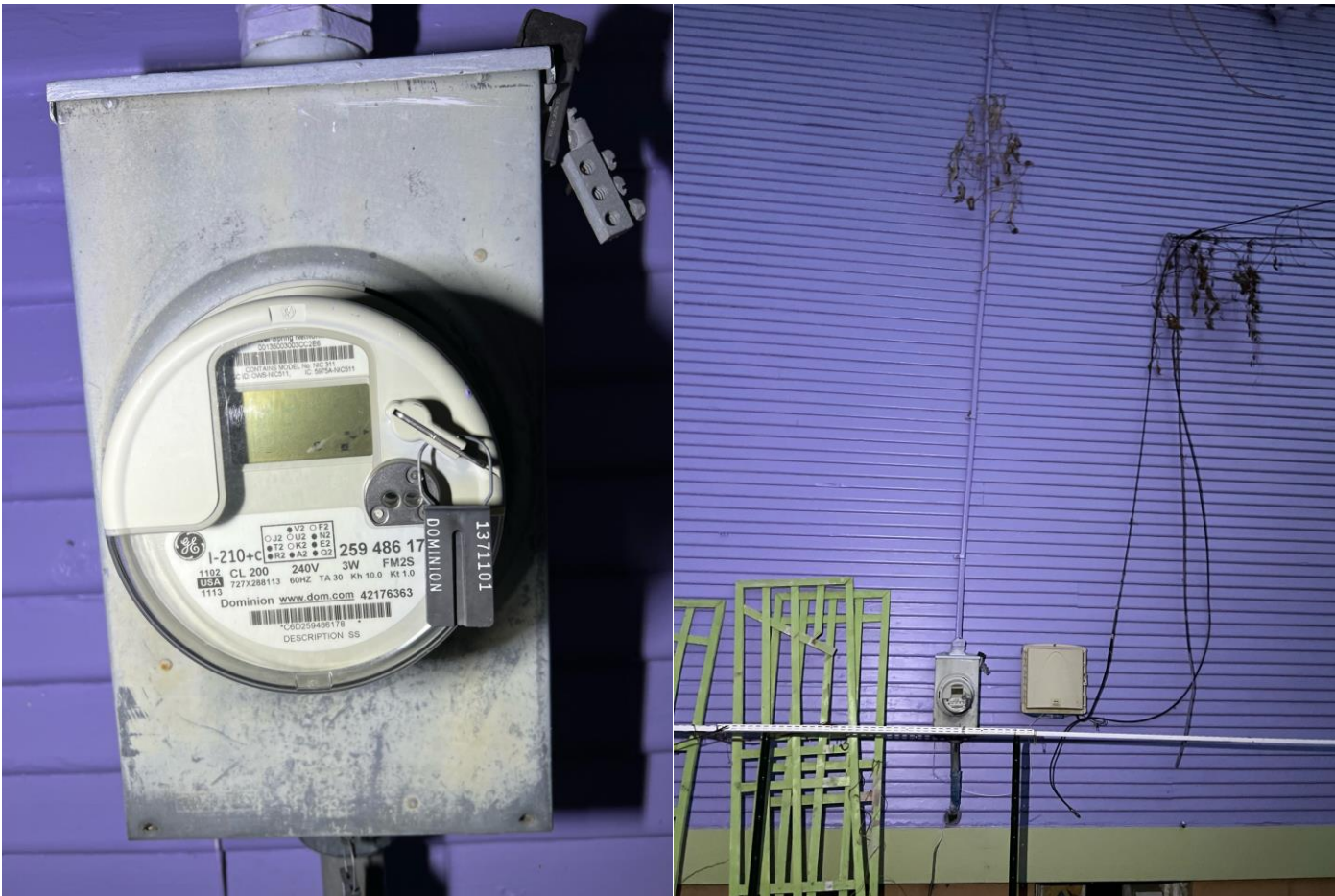
Figure 8 & 9: Meter is mounted on left side of the house. We will be able to place disconnect and load center near this one.
