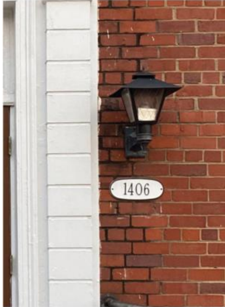
/ EXISTING LIGHT FIXTURE
