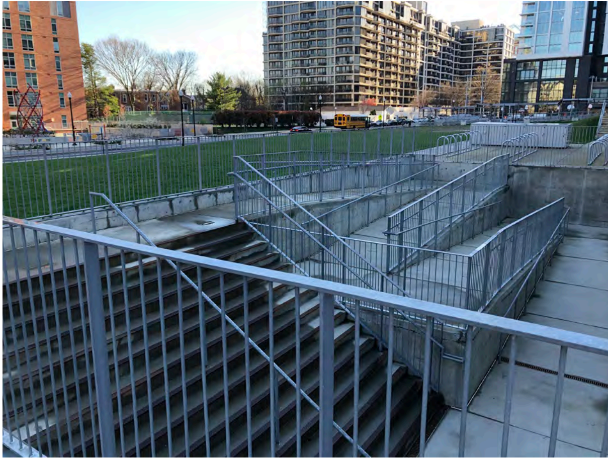
Temporary Stair and Ramp to Heights Building G1 Level (Shriver Administrative Area)
