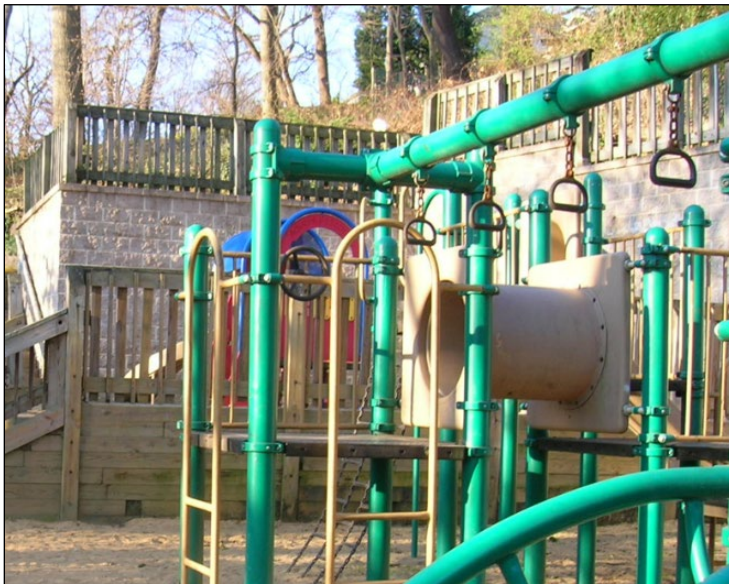
Figure 4: The retaining walls alongside the playground in Cherrydale Park, which must have safety handrails installed at the top as a requirement of the VUSBC (Source: DPR)
