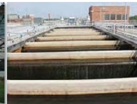
Water Pollution Control Plant
