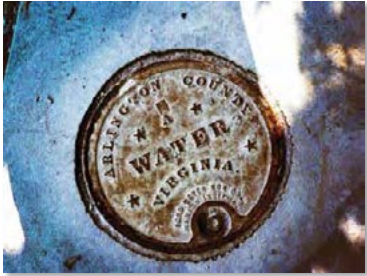
Residential Water Meter
