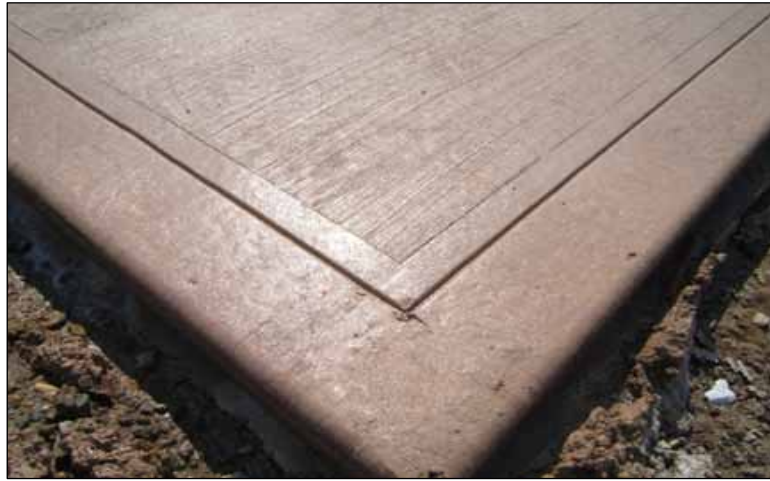
FIGURE 3. Example of Acceptable Clear Zone Treatment (broom finish) Detail of broom finish texture. Note the 2" troweled edge inside the tooled joint.
