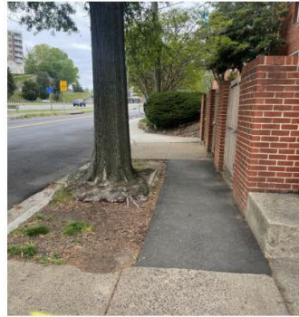
C FAIRFAX DRIVE SIDEWALK: +/-5' WIDE; LARGE STREET TREES IN POOR CONDITIONS
