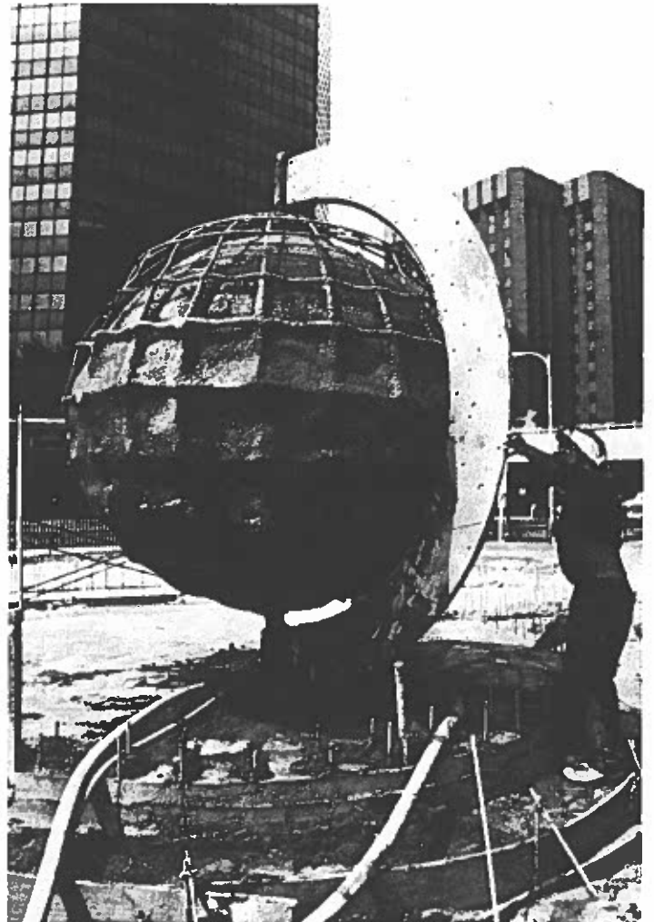
Bottom photograph shows construction of a gunite sphere using the semi-circular screed
