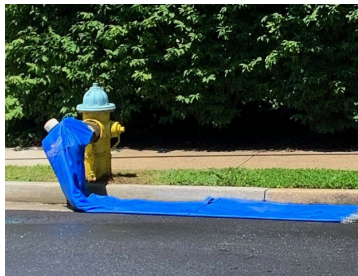
Fire hydrants are flushed every spring as part of the disinfectant switch in the water distribution system.
