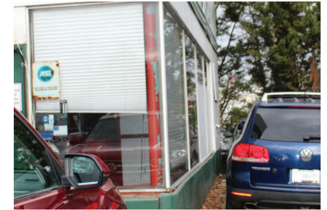
Figure 014 Plate glass window. EHT Tracerics, December 2018.
