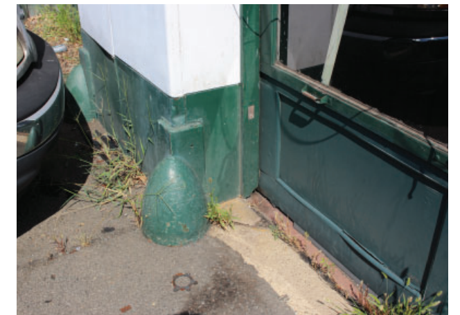
Figure 016 Corner bumper guards at garage bay entrance. EHT Tracerics, August 2019.
