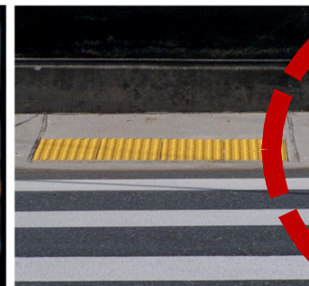
Detectable Warning Strip
