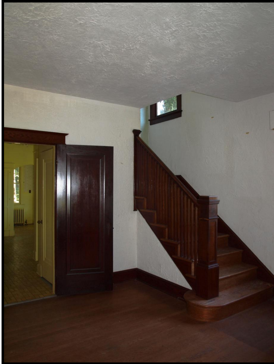
Photo 13: Interior view from the front door, facing northwest. Note the original American Chestnut woodwork and trim, and the pulled plaster wall finish.
