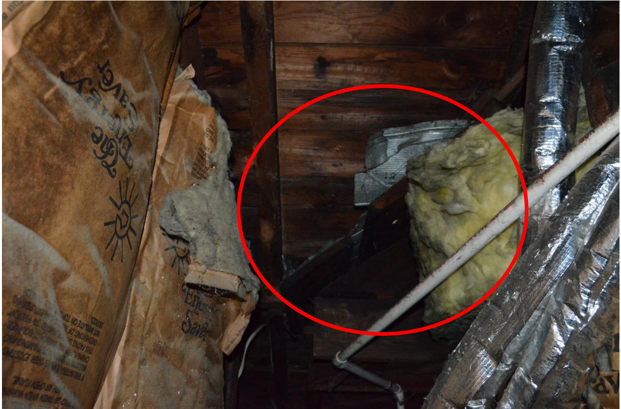
Figure 14: View of remaining parts of the I-house's western slope of its side gabled roof with metal shingles still attached. The shingles are circled in red.
