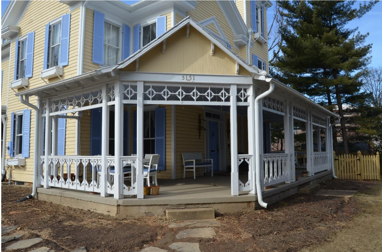
Figure 2: View of the wraparound front porch. Note the “gingerbread-styled” balustrade, chamfered wood posts, pierced frieze, and decorative wood brackets.
