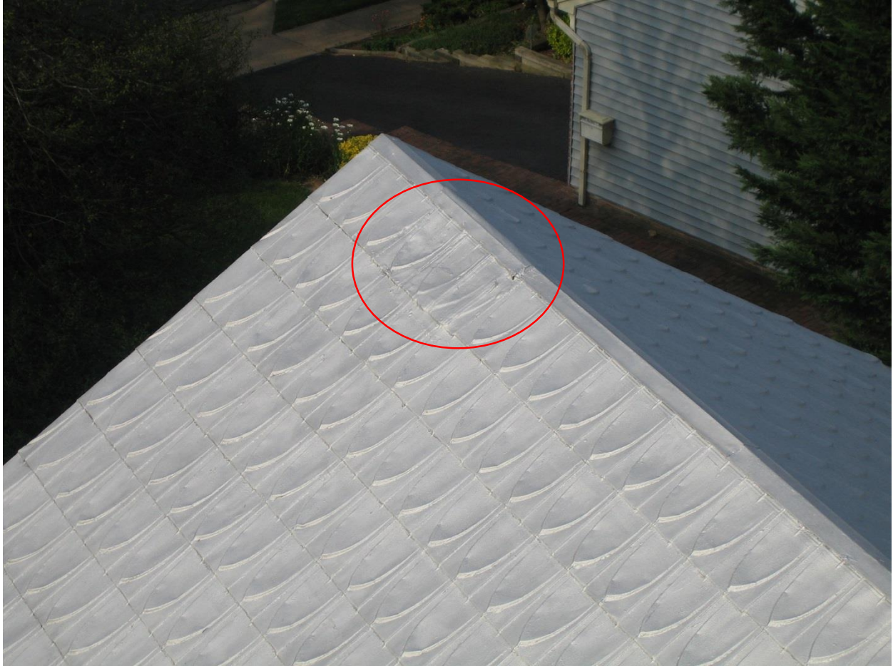
Figure 9: View of the southern end of the original I-house's roof. The location of the original chimney is circled in red.
