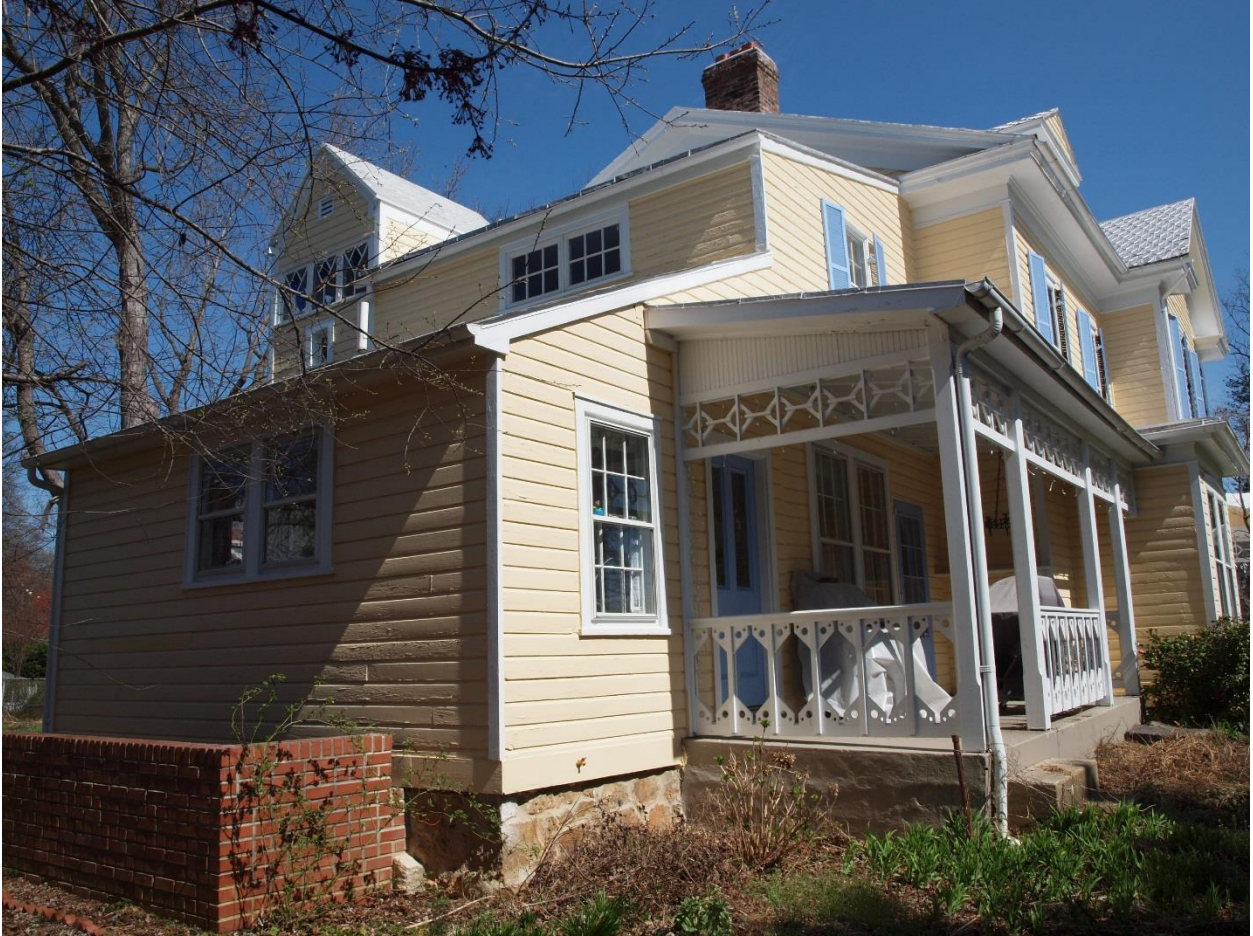
Figure 5: View of the south and west elevations looking northeast from subject property.
