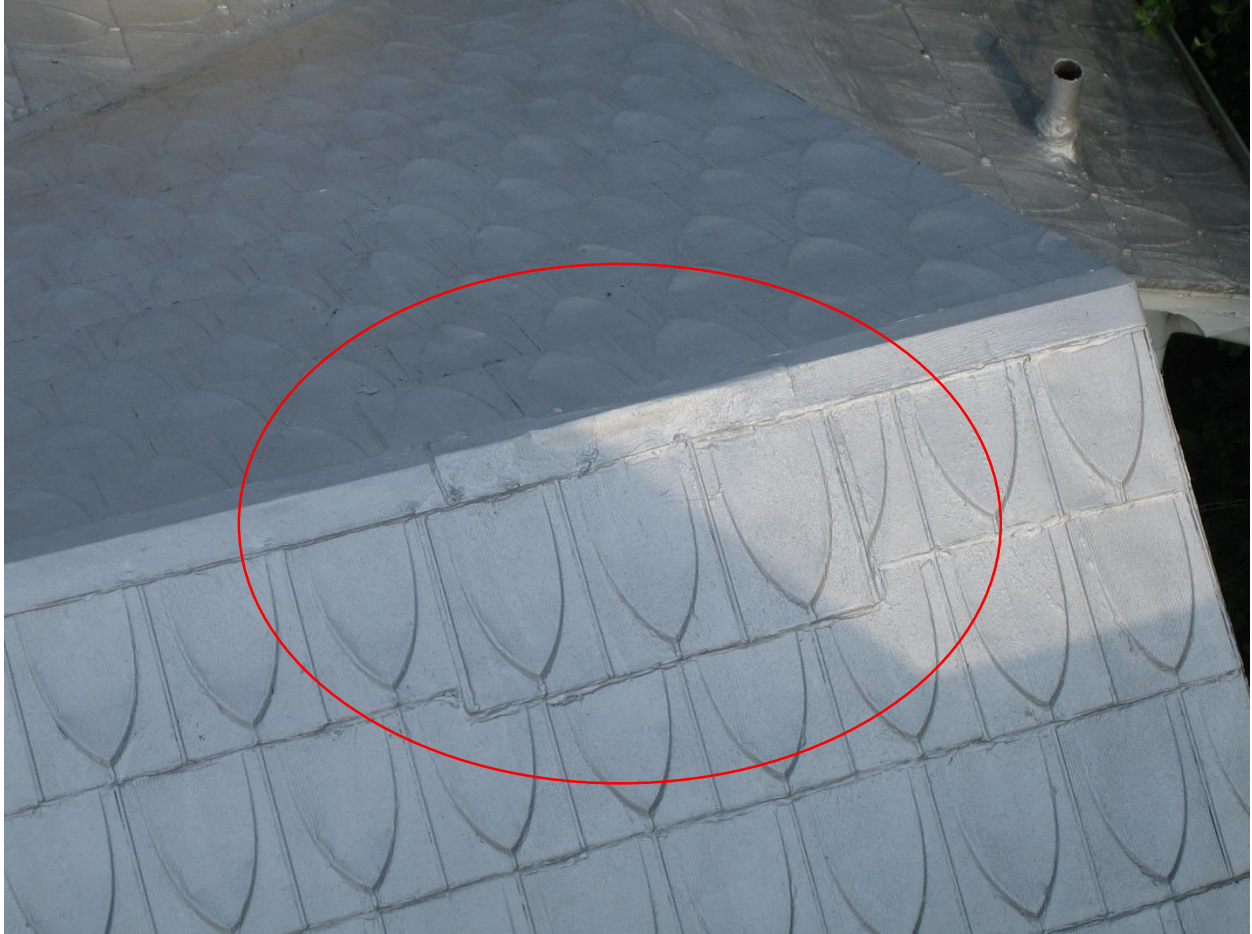
Figure 10: View of the northern end of the original I-house's roof. The location of the original chimney are is circled in red.
