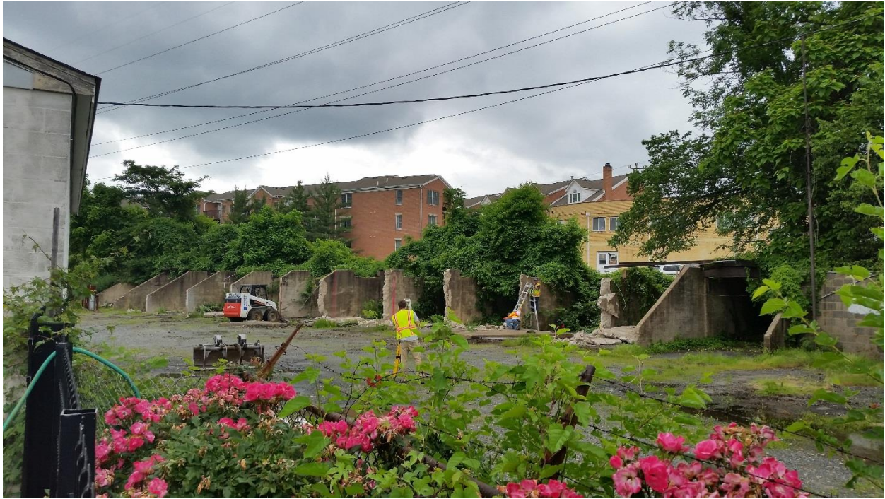
Figure 31: Active demolition of Benjamin Elliott's Coal Trestle, looking northwest near Lee Highway. The pink lines on the concrete piers represent the property boundary and the extent of demolition of the trestle. Source: Arlington County Historic Preservation Program Staff, June 5, 2014.
