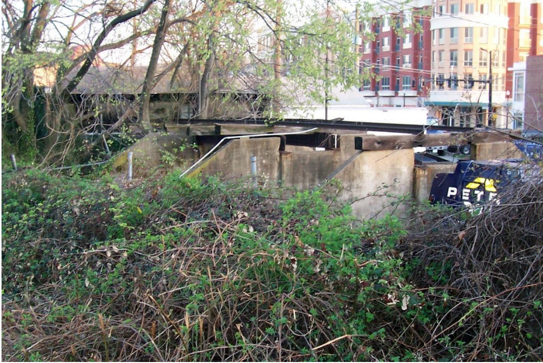
Figure 30: “Overgrown W&OD Railroad Trestle, Arlington, Virginia,” 2007. Looking from the W&OD Trail towards the remaining rails and ties at the east end of the coal trestle.
