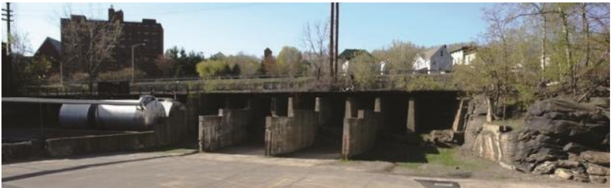
Figure 9: A combination trestle and ground storage bin in Little Falls, New York. The design and concept is very similar to Elliott's coal trestle. The concrete piers also served as storage bins that separated the different sizes of coal.
