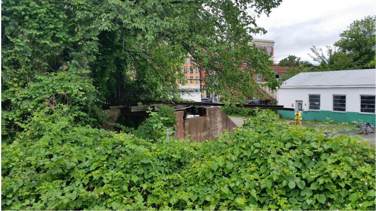
Figure 32: Active demolition of Benjamin Elliott's Coal Trestle, looking southeast from the W&OD Trail. The pink lines on the concrete piers represent the property boundary and the extent of demolition of the trestle. The above tracks were salvaged and conveyed to the NVRPA.
